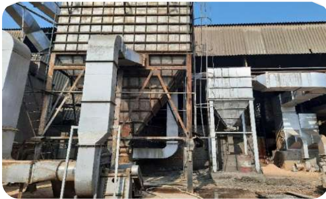
Thermic Fluid Heater
