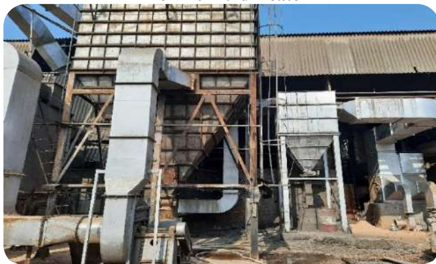
Thermic Fluid Heater
