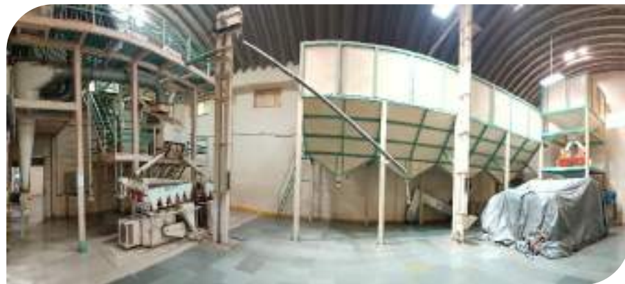
Navrang Cleaning Plant
