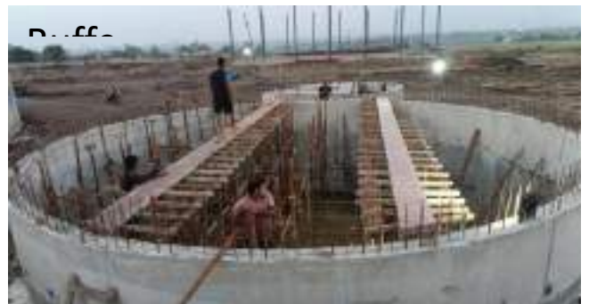
Buffer Tank (Ariel View)
