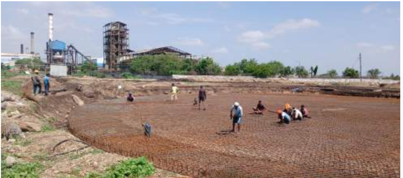
Compressed Bio Gas (CBG) Digester Raft
