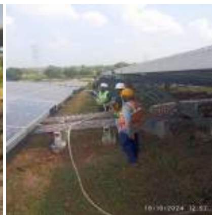
Solar Module Cleaning
