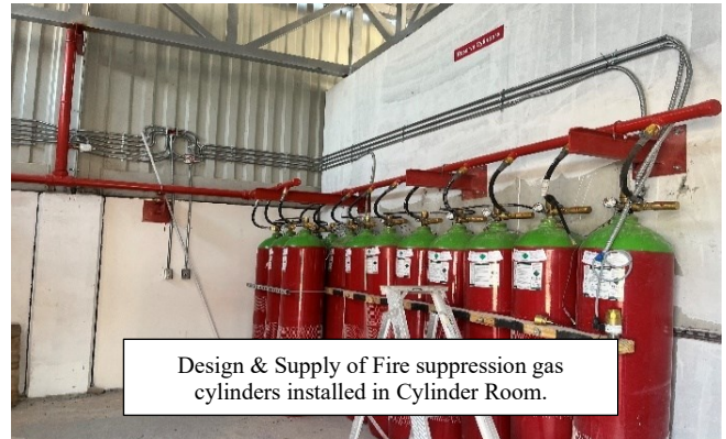
Gas Suppression System
